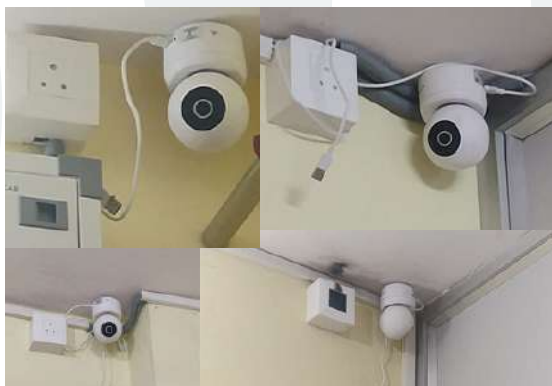
Four CCTV Cameras
